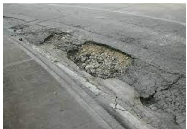
Pot holes can also damage cars and cause crashes.
